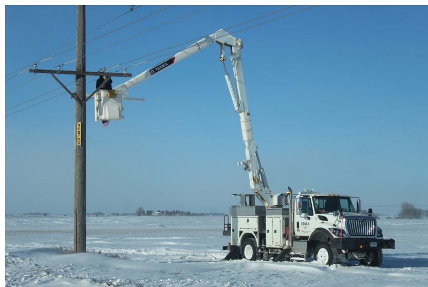
BENCO line crews worked to restore power during cold, winter weather conditions near Minnesota Lake in December 2020.
